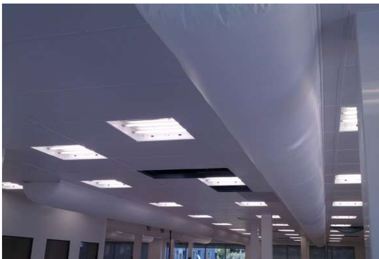
Semi-circular 100% duct inside offices
